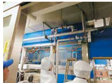
Energy saving diagnosis of factory facilities
